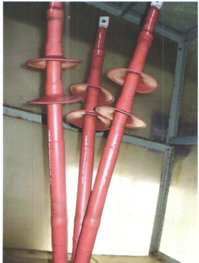
Photograph No.2: Terminations after Humidity Test
