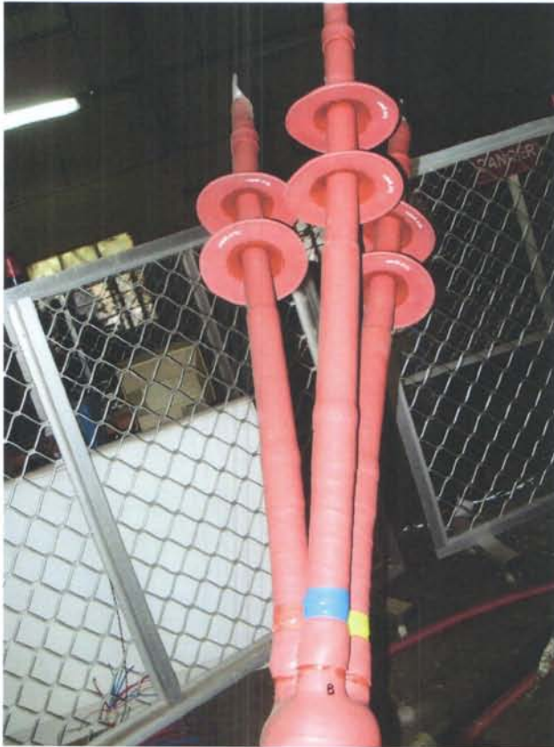
Photograph No.1: Terminations before Humidity Test
